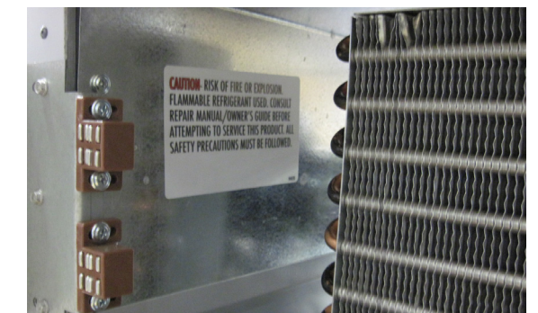
CONDENSING UNIT AREA SIDEWALL
